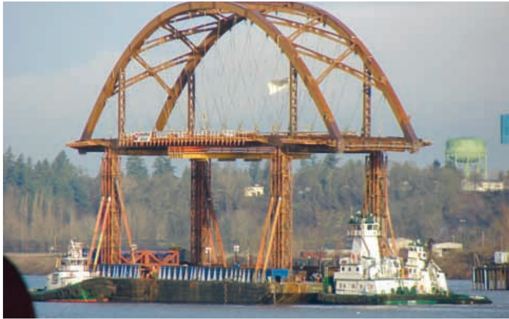
With good weather and smooth water, four Foss tugs move Portland's new Sauvie Island Bridge up the Multnomah Channel. The tugs, from left, are the Daniel Foss , PJ Brix and Jim Moore . The Betsy L is out of sight on the other side of the barge.
